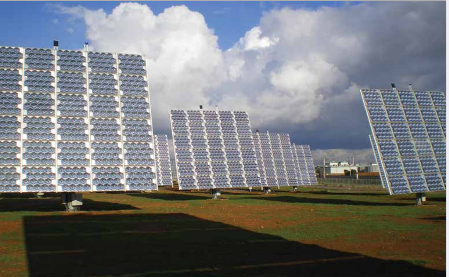
One of the CPV plants located at ISFOC headquarters
